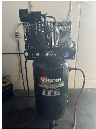
Sanborn Vertical Drum Air Compressor
